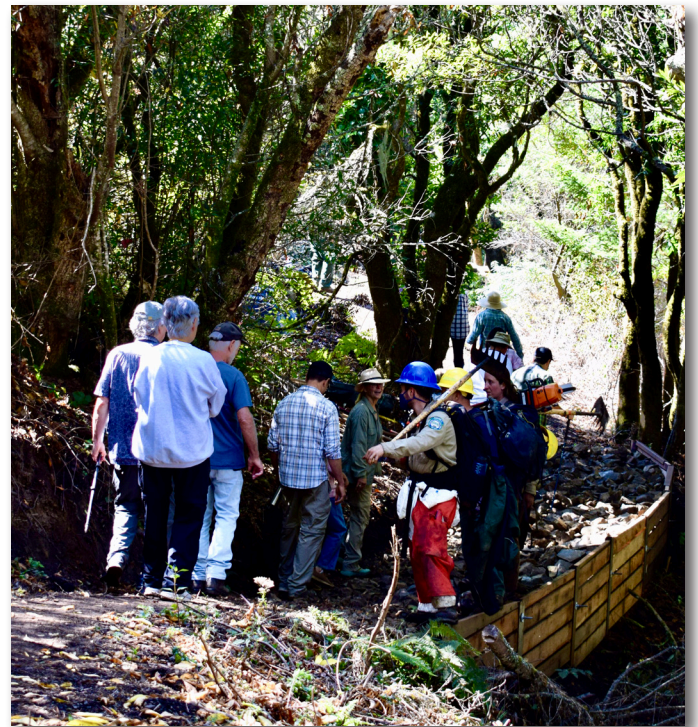
Rebuilding the State Parks trail near Redwood Creek—moving it up and out of the wetland..
