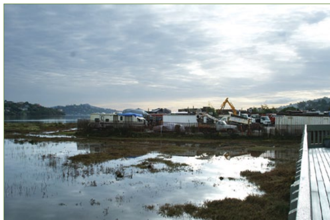
The Whalers Point site is on Richardson Bay between Sausalito and Mill Valley, behind the outdoor teak dealer.
