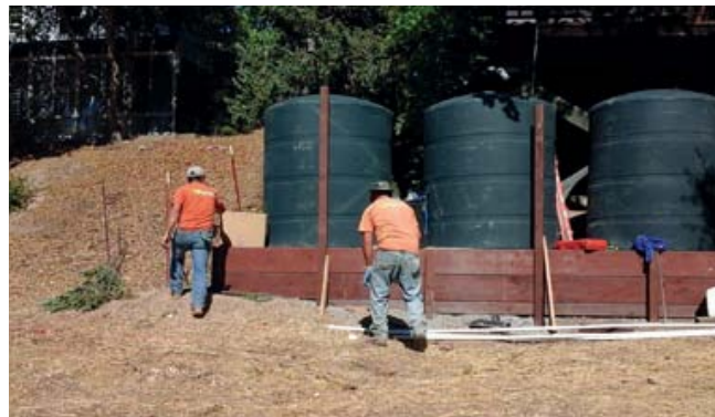
An Equinox crew installs Rainwater Harvesting Tanks that connect directly to an existing drip irrigation system.
